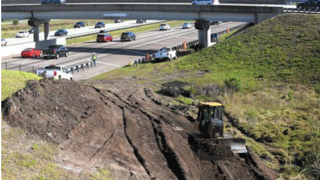
Construction is beginning on the I-4 Ultimate project with earth removal at the Maitland interchange originally put there to help fill a sinkhole. April 10, 2015. (George Skene, Orlando Sentinel)
