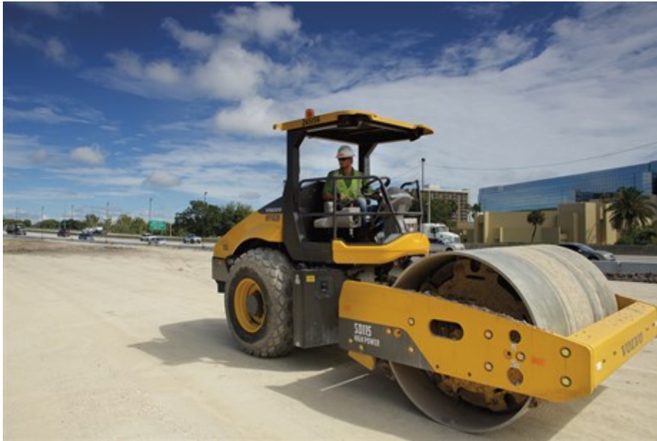
The Volvo SD115 soil compactor is carrying out important duties on the project
