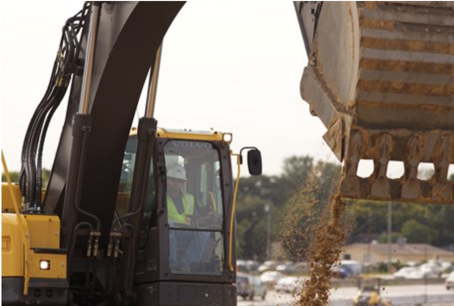
Good visibility from the excavator cab is highly important for the work
