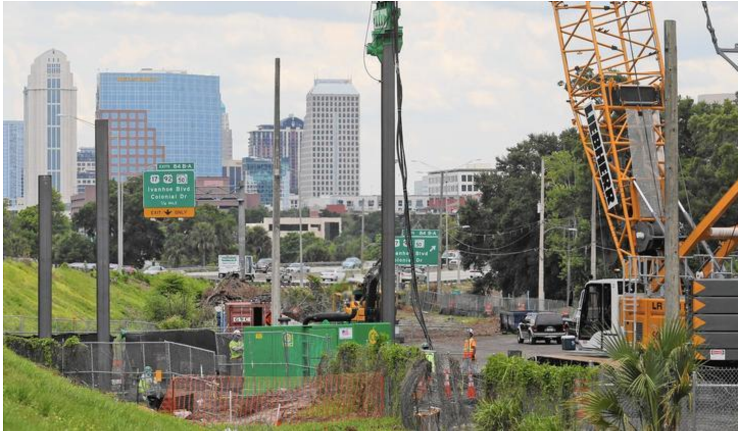
CAPTION Red Huber, Orlando Sentinel Work crews for the I-4 Ultimate Project drive steel pilings Tuesday, June 9, 2015 at Interstate 4 and New Hampshire St. Crews assembled $80 million worth of heavy equipment and machinery up and down the 21-mile stretch of Interstate 4 that is going to be rebuilt. Included in the armada: : 250+ pickups, 30+ cranes, 40+ Front end loaders, 30+ Dozers, 30+ Rollers, 30+ excavators and 9 massive German-made Liebherr Crawler cranes with up to 200-ton lifting capacities. (Red Huber/Staff Photographer)
